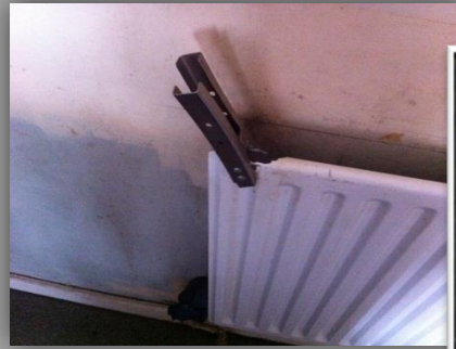
BEFORE: A clamp to stop the radiator from leaking!
